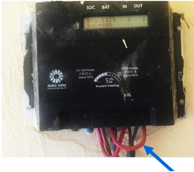
Figure 4. A faulty charge regulator in Rubaya health center has been bridged (see arrow).
